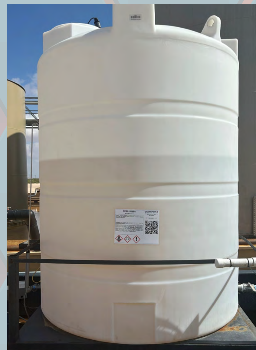
Picture 2: Shows chemical storage tank with updated label that has QR-code linked to the product SDS.
